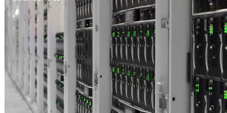
South Pole Group delivers GoldPower for SAP data centres
