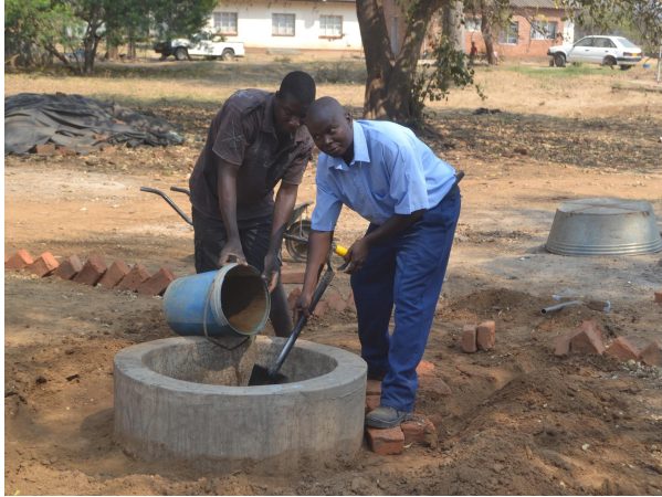
The Chitsungu Hospital biodigester is now operational, Mbire District
